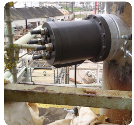
OD nozzle test pictured above was accomplished on a 2", 300#, nozzle on a 16" propane line; the test utilized inflatable seal technology to perform a localized hydro test of the full penetration weld on the 16" pipe
